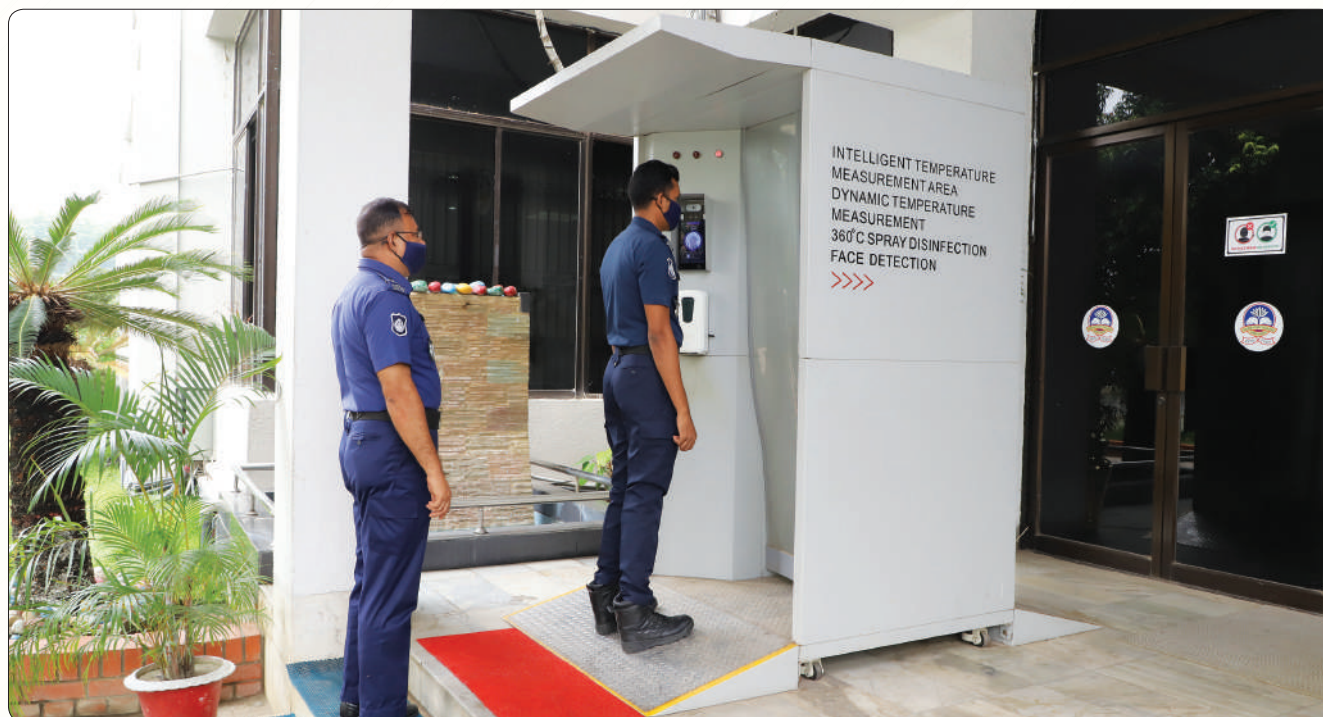
Smart Temperature Measurement system installed at entrance
